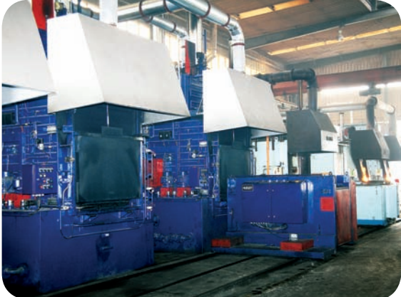
Furnaces for heat treatment process
